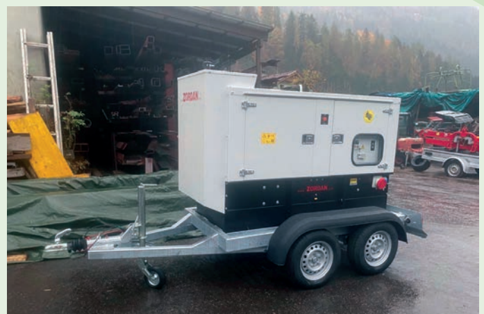
Neues mobiles 80-KVA-Notstromaggregat
